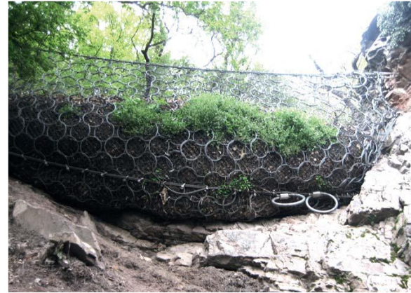
Flexible barrier (GEOBRUGG, Lorch, Germany)
