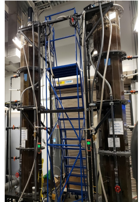
Sequencing Batch Reactors (SBRs)
