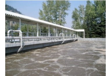
water treatment and recycle
