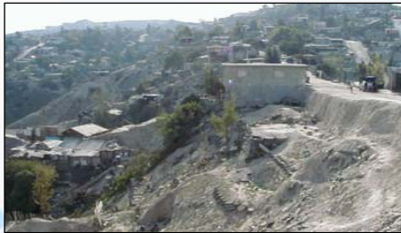
Slope stability improvement in a Mexican township using terraces of used tires
